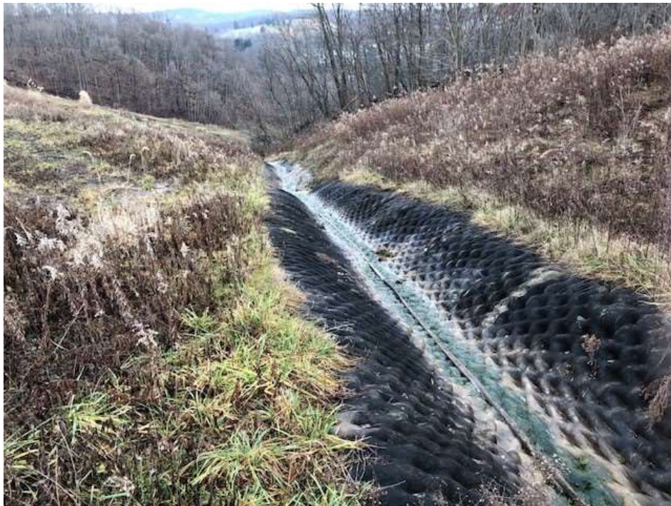
Photograph 12: Eastern view of south revetment matt lined stormwater channel on east landfill slope.
