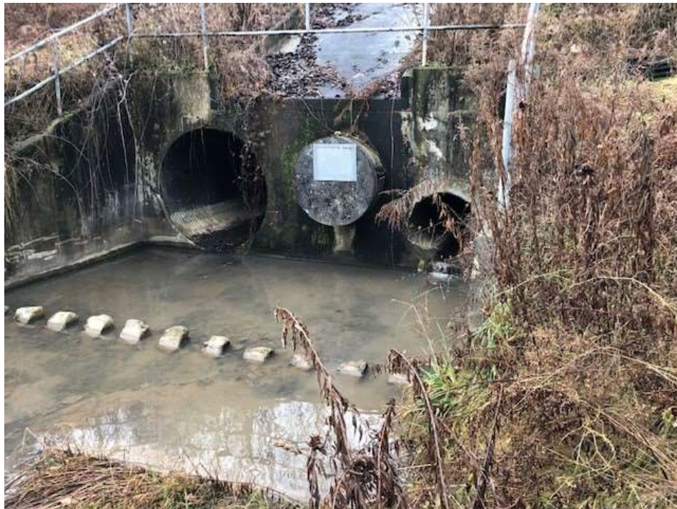
Photograph 21: View of Sedimentation Pond emergency spillway outlet, non-contact stormwater outlet pipes, and capped contact stormwater (leachate) pipe. Contact stormwater drains to pump station.
