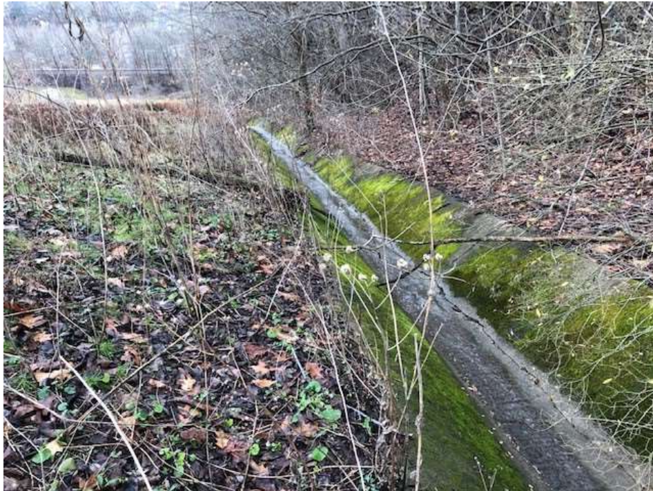
Photograph 14: Eastern view of south concrete lined stormwater channel on east landfill slope.
