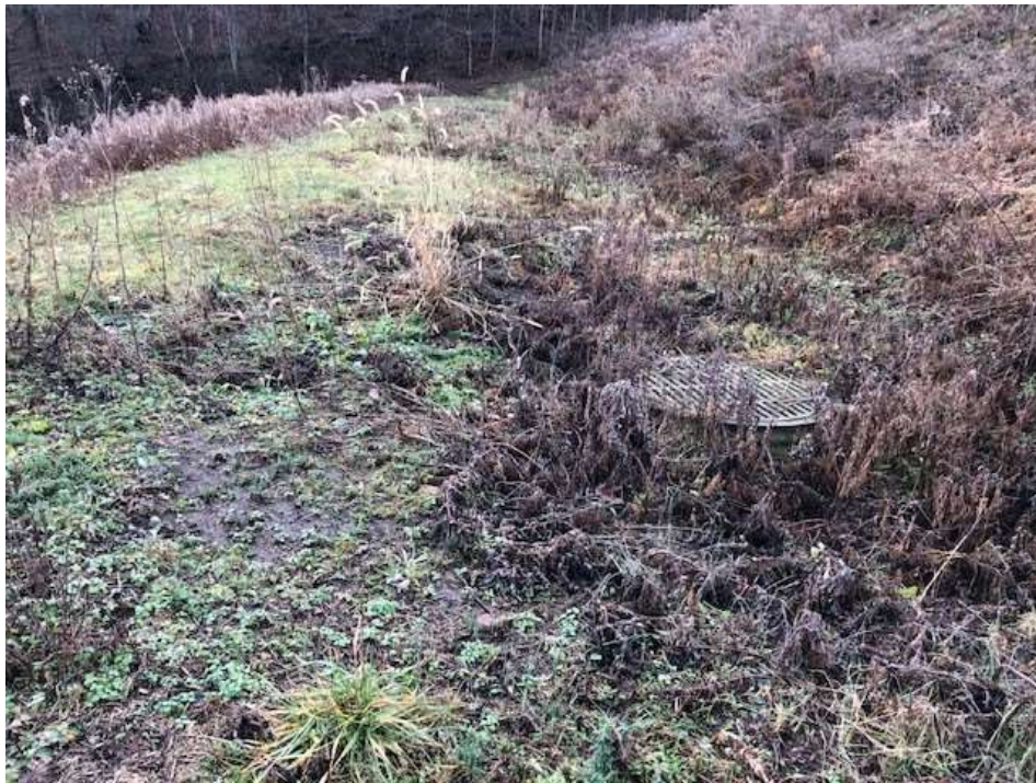
Photograph 15: South view of mid-slope bench and non-contact stormwater inlet on east landfill slope. Vegetation is established with no indications of stability issues.
