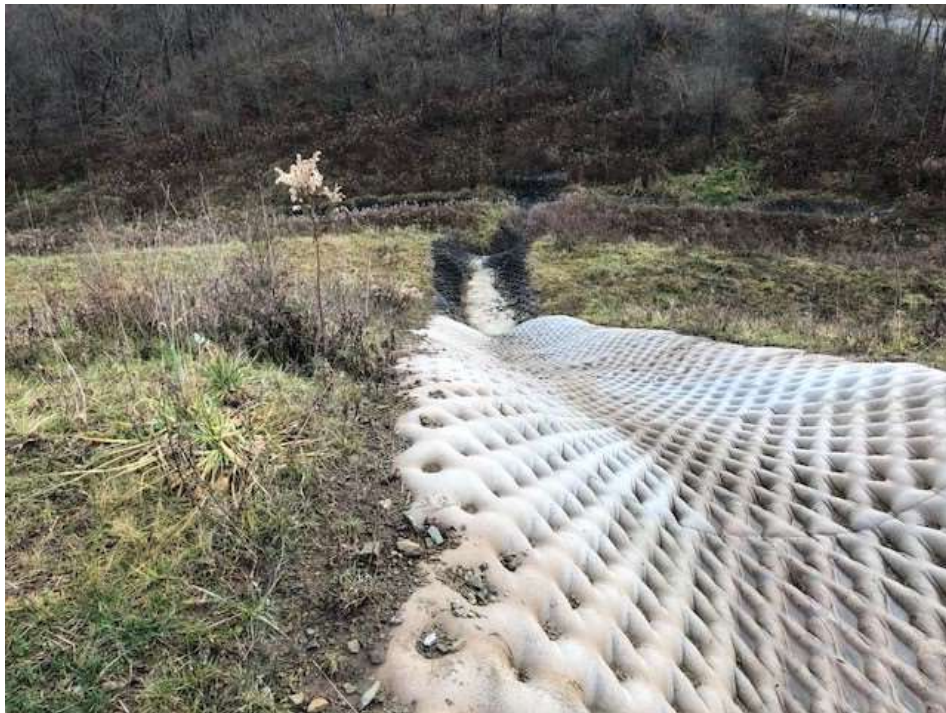
Photograph 10: View of revetment mat lined stormwater channel installed in 2020 at south end of upper bench on east landfill slope.
