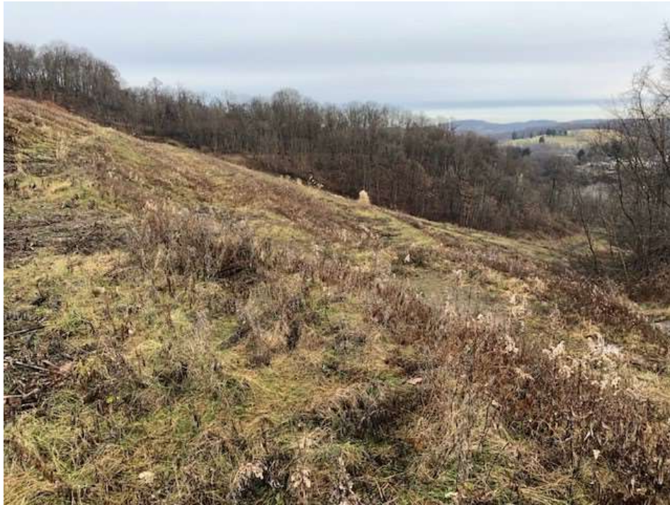
Photograph 13: North view of upper east landfill slope. Vegetation is established. Benches have been mowed. Woody vegetation has been cut. No indications of stability issues.
