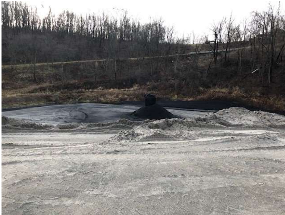
Photograph 7: View of contact water (leachate) riser located in southwest corner of landfill.
