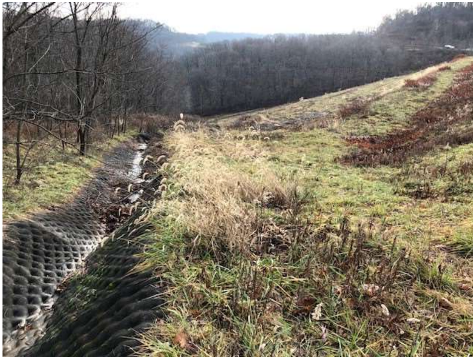
Photograph 11: Eastern view of north revetment matt lined stormwater channel on east landfill slope.
